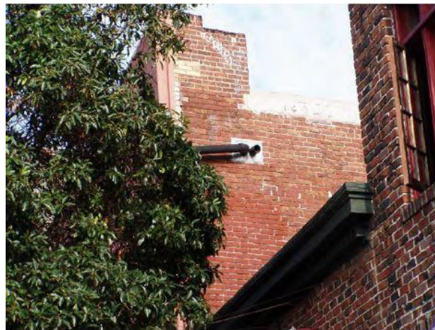
Brick upper south wall near front façade viewed facing north (photo by JRP Historical Consulting, 2004).
