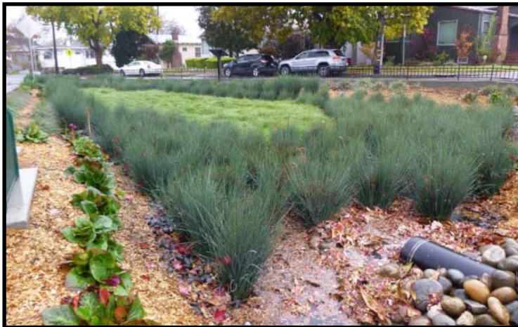
Concrete traffic island reconstructed with a bioretention facility at Rose and Hopkins Street
