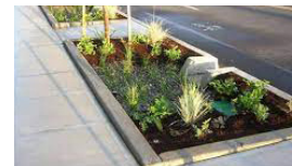
Stormwater Planter Box
