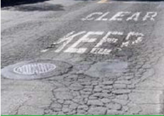
Street surface in need of repairs
