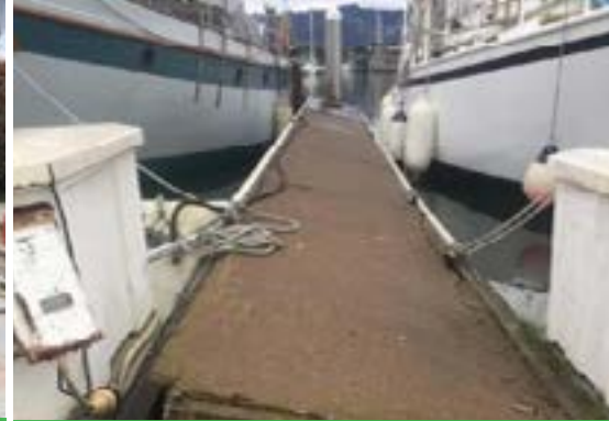
Marina dock in need of repairs
