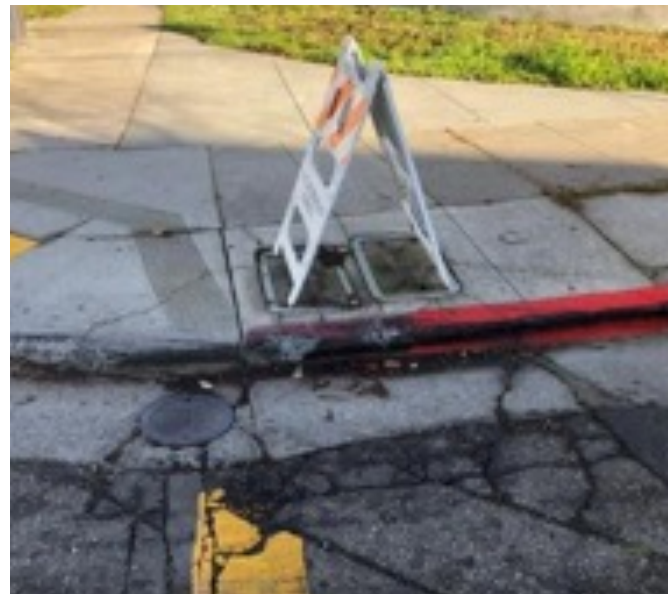
Sidewalk tripping hazard
