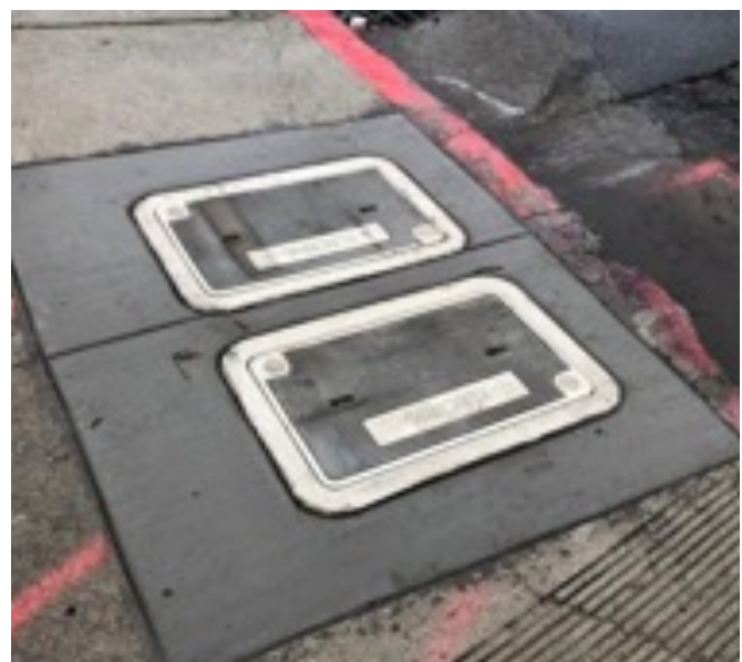
Sidewalk hazard repaired
