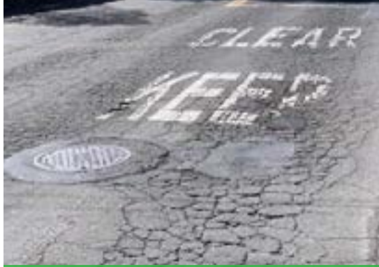
Street surface in need of repairs
