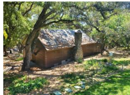
Scout Hut in 2022 with recent irrigation improvements at the upper area of park in foreground.
