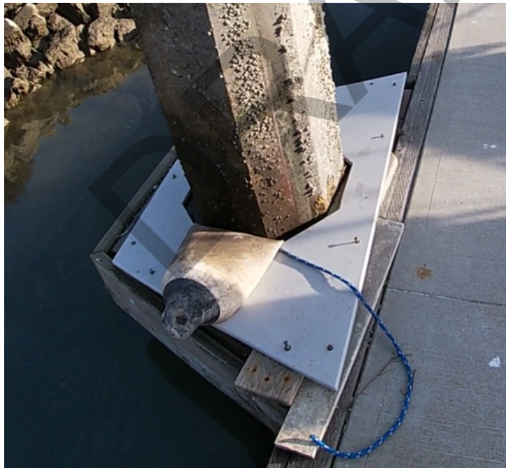
Damaged guide at I Dock. It appears the buoy is acting as a temporary replacement for rub strips
