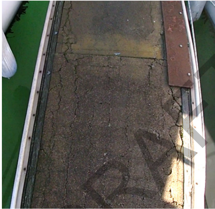
Delaminated finger between slips 139 and 141. The cracking on the walking surface is typical of delamination.
