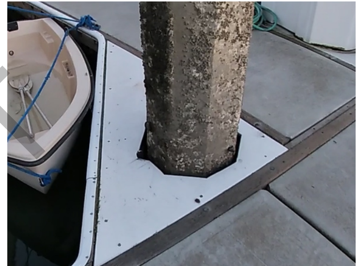
Pile guide hidden beneath polymer cover board
