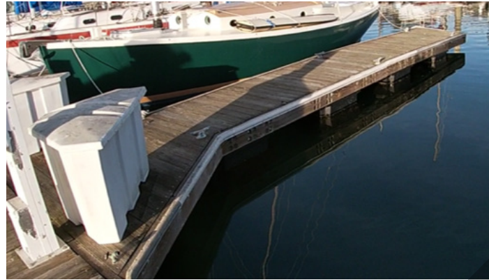
Twisted finger at F Dock. Note the middle section of the finger is slightly raised in comparison to the ends
