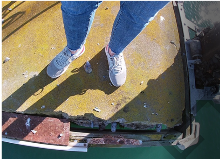
Typical cracking and spalling at finger ends. Note the cracking occurs on the perimeter of the concrete float module
