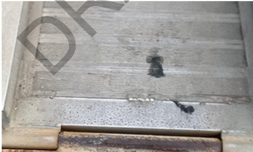
Corroding hinge at the top of the non-ADA accessible gangway.
