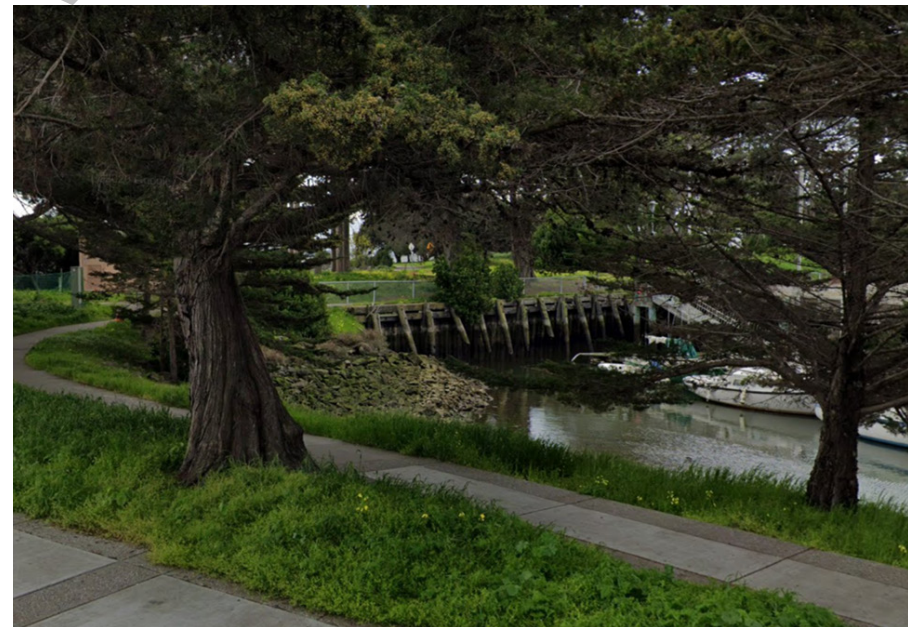
Revetment at the old boat launch facility. Note the crest elevation and top of bank elevation do not match.
