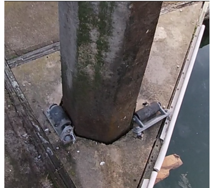
Internal pile guide. Note the unattached pile roller assembly, allowing the pile to make direct contact with the plywood
