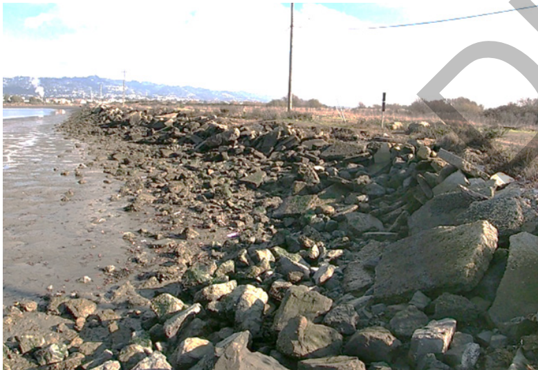
Low elevation area at the shoreline where Marina Blvd meets Virginia St Ext
