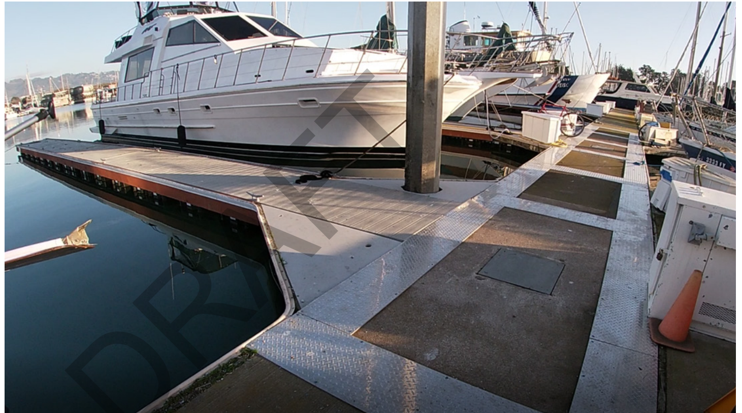
Diamond plate sheet covers and a newly replaced finger along O Dock's eastern edge.
