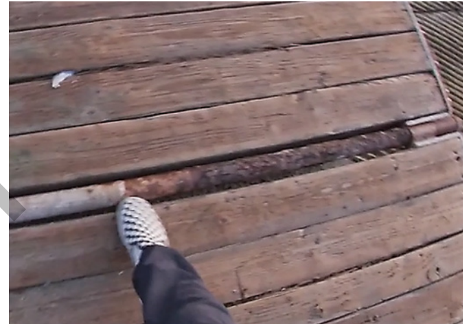
Corroding hinge between boarding float modules
