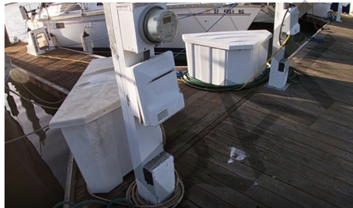
Typical utility configuration at F Dock
