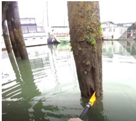
Damaged pile beneath the G and H Dock restroom
