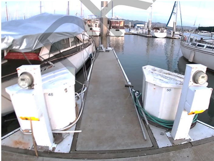
Typical utility configuration at B and C Docks
