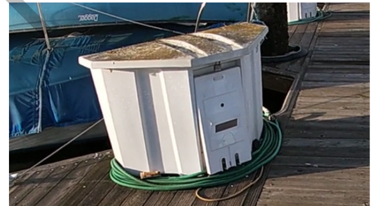
Typical utility configuration at G Dock
