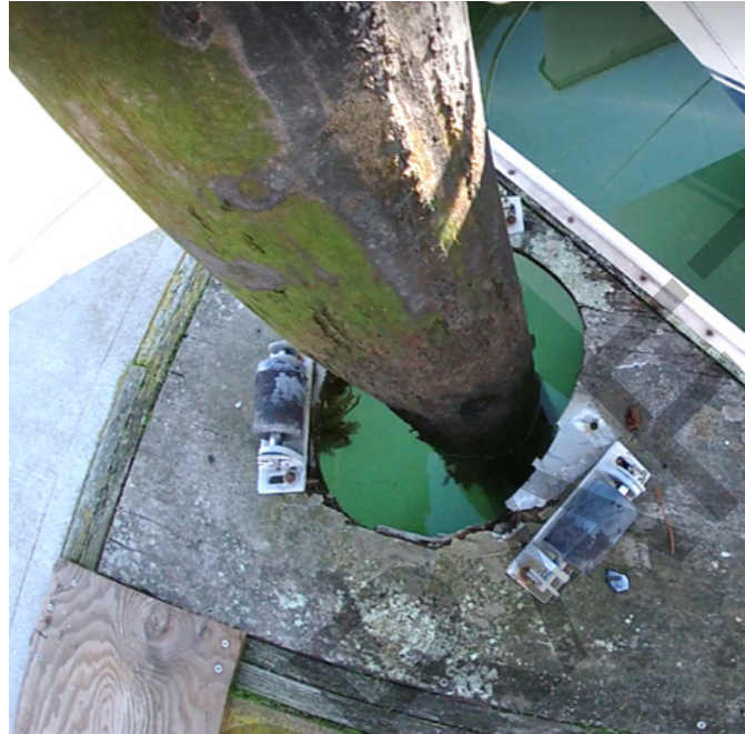
Damaged internal pile guide. Note the unattached pile roller assemblies and widening hole in the plywood
