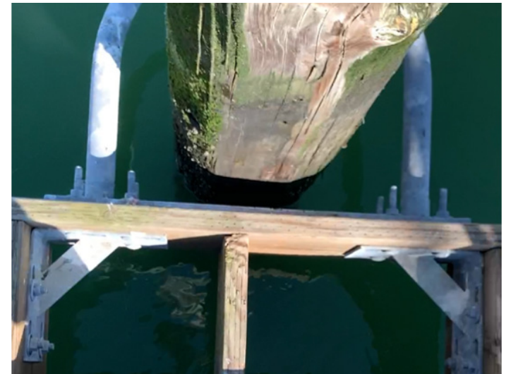
Exposed finger end revealing construction method for the docks
