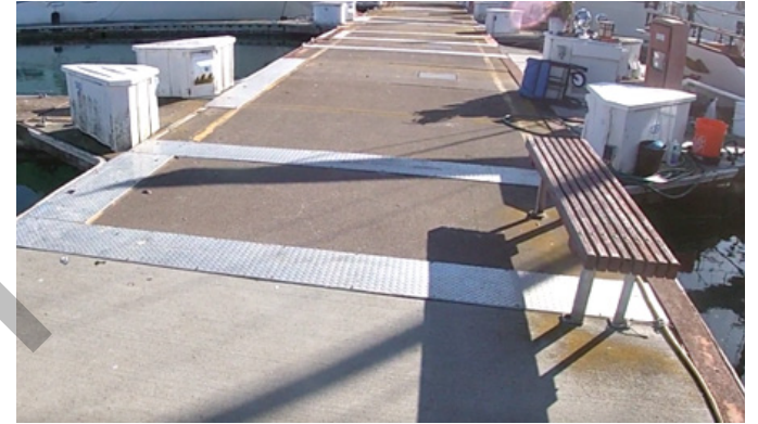
Diamond plate covers at the edges of the floats. Covers hide cracks and tripping hazards
