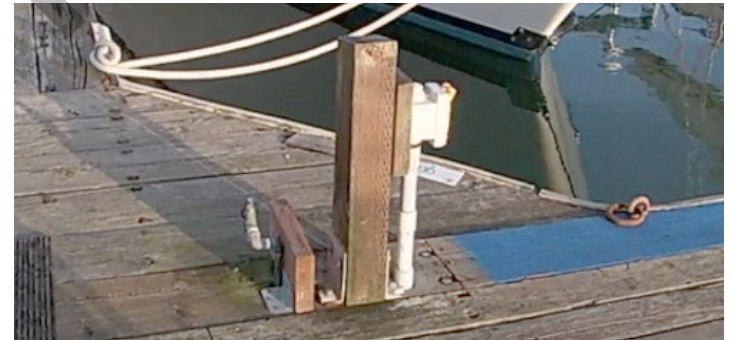
Typical power and water utilities at D and E Docks
