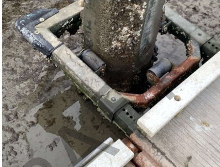
Corroding steel hinge and pile guide
