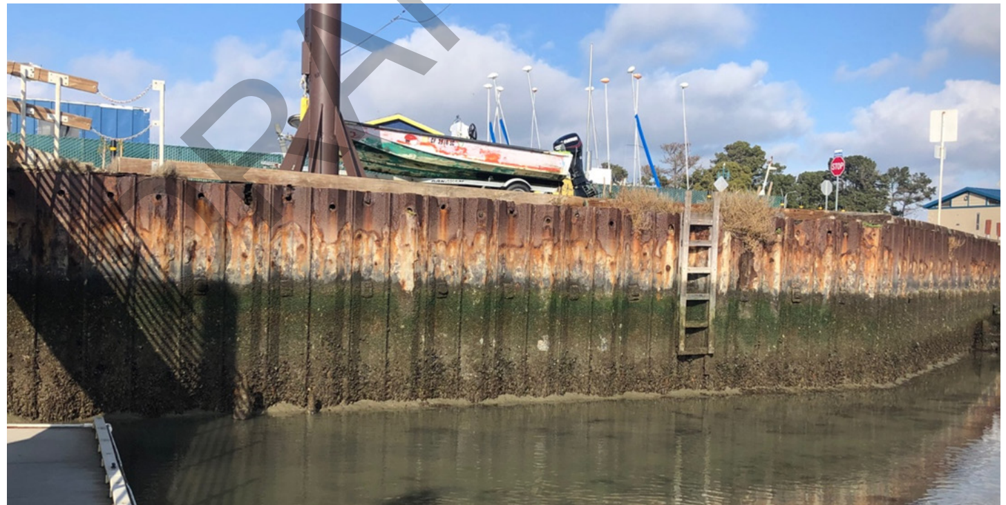
South Sailing Cove Seawall. Note the heavily corroded steel of the sheet piles.
