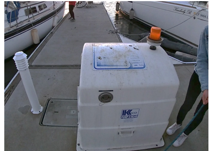
Keco sewage pumpout and auxiliary connection in the distance
