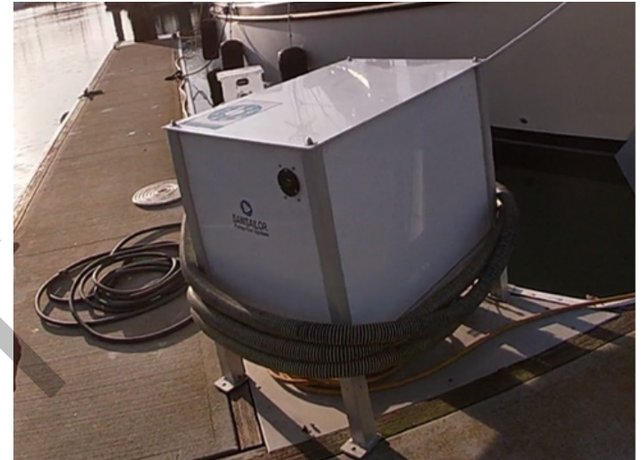
Sanisailor sewage pumpout at I Dock
