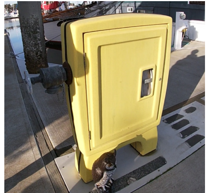
Typical fire cabinet with fire water access
