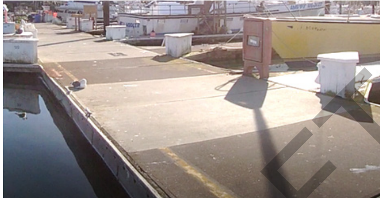
Main walkway of K Dock. Note the width of the dock as well as the different color of the float modules. Floats lighter in color are likely replacements
