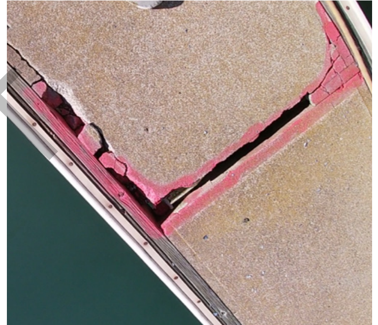
Typical cracking at edges of concrete float module
