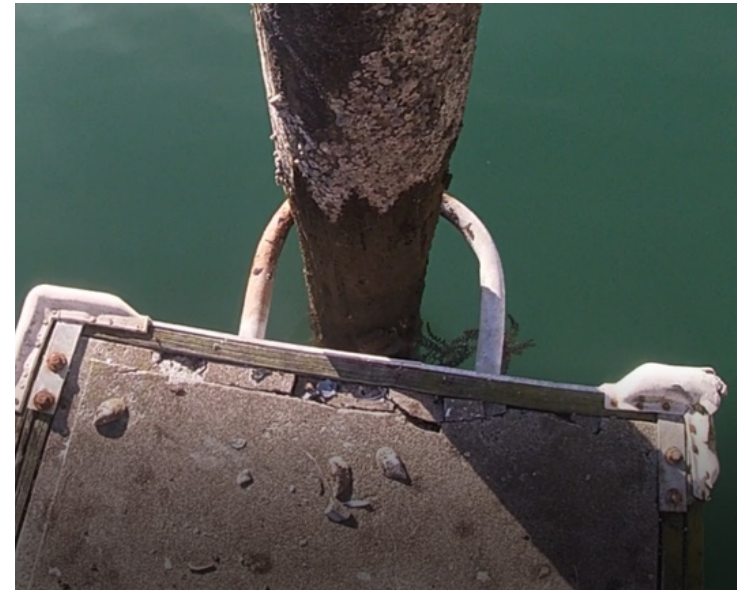
Cracking concrete and finger end
