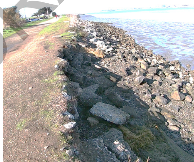
Typical scarp in revetment slope
