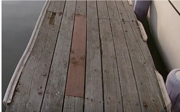
Typical timber deck at D and E Docks. Notice the replaced plank with a redder hue
