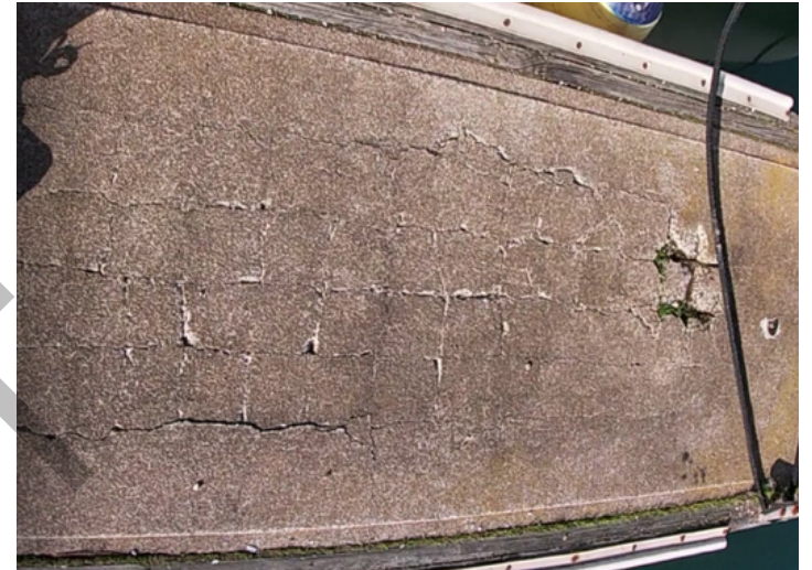
Delamination of the concrete dock module. This damage is typically covered by plywood or steel and is not visible
