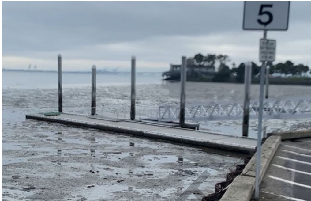
Photograph 2: Middle Dock Grounded at South Sailing Basin at 0' MLLW.
