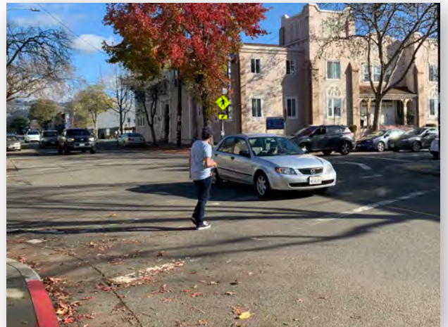
Alcatraz Avenue at King Street. Faded crosswalk markings decrease pedestrian visibility and awareness.
