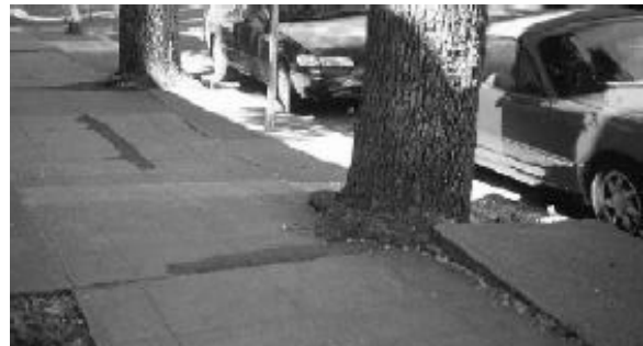
Repair sidewalk cracks and uplifts from tree roots in a timely manner
