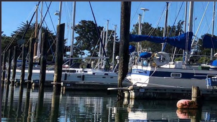
Decaying Timber Piles
