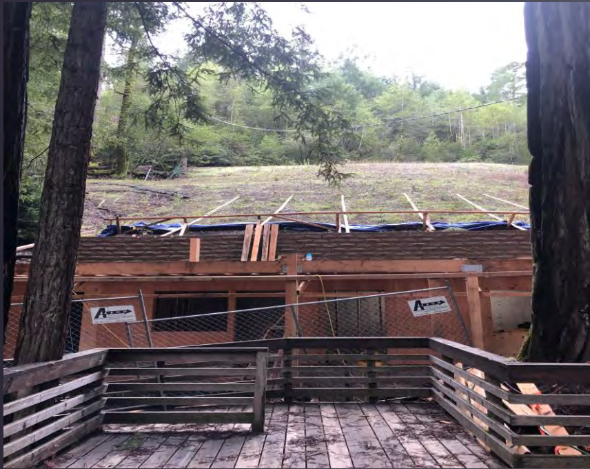
Cazadero Camp Jensen Dormitory with landslide fix in background
