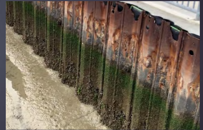
Aged Sheet Pile Wall – South Cove
