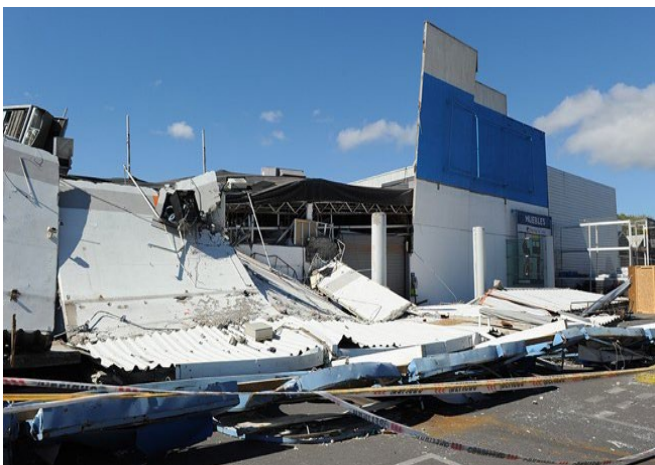
Partial collapse of a tilt-up building with insufficient roof-wall connections during 2010 Chile earthquake
