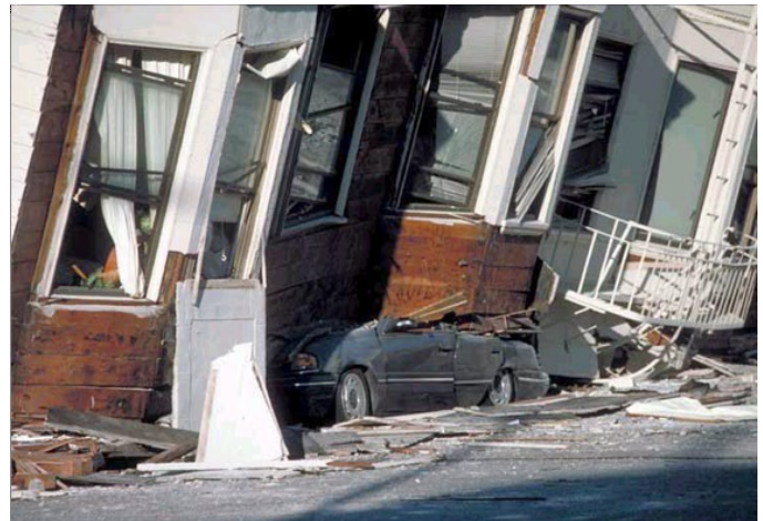
Soft Story destroyed by 1989 Loma Prieta earthquake
