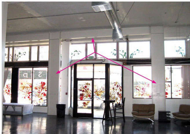
Retrofit of a retail storefront using a steel moment frame at the interior
