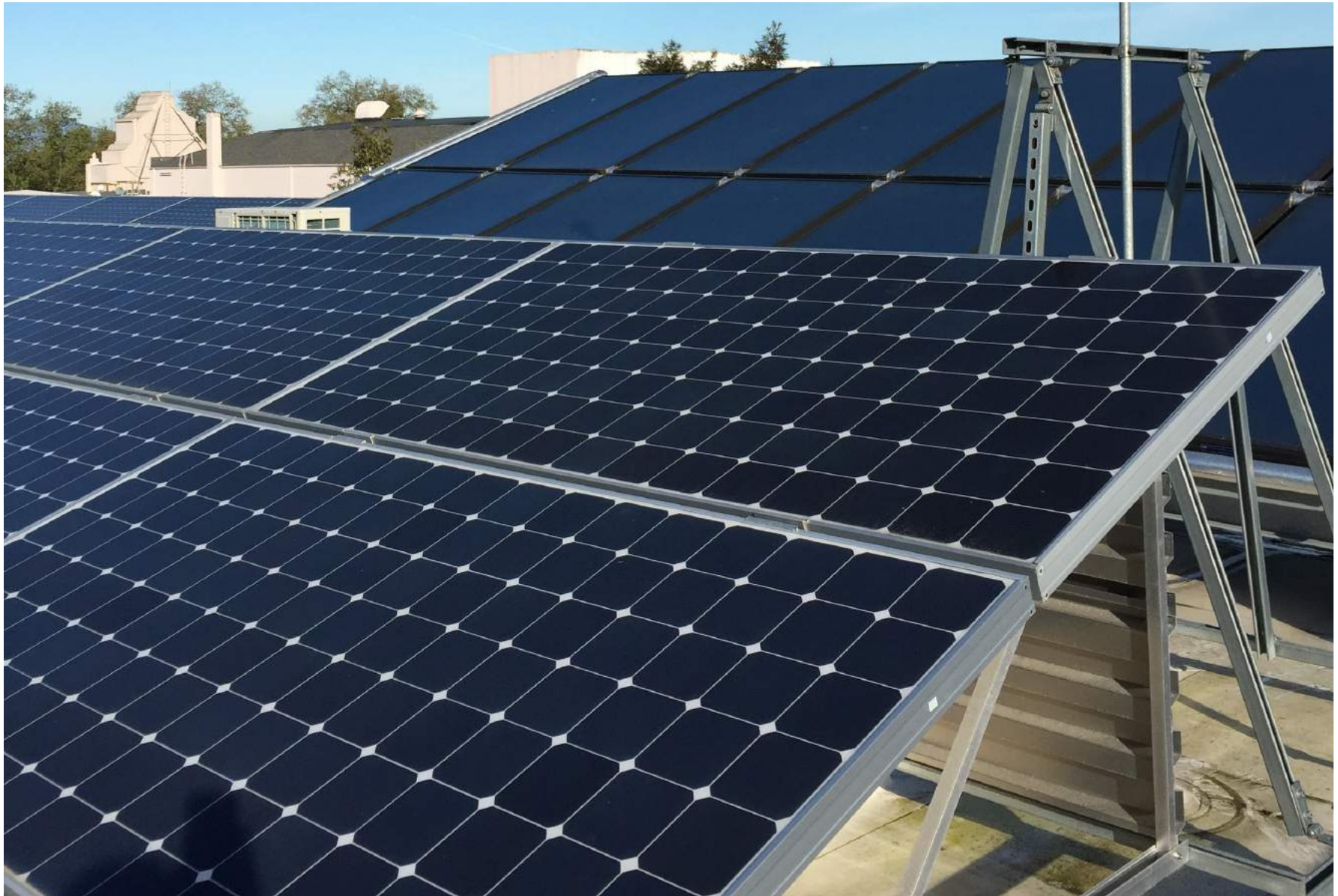
Solar panel array on the rooftop of the Zero Net Energy West Branch Berkeley Public Library
