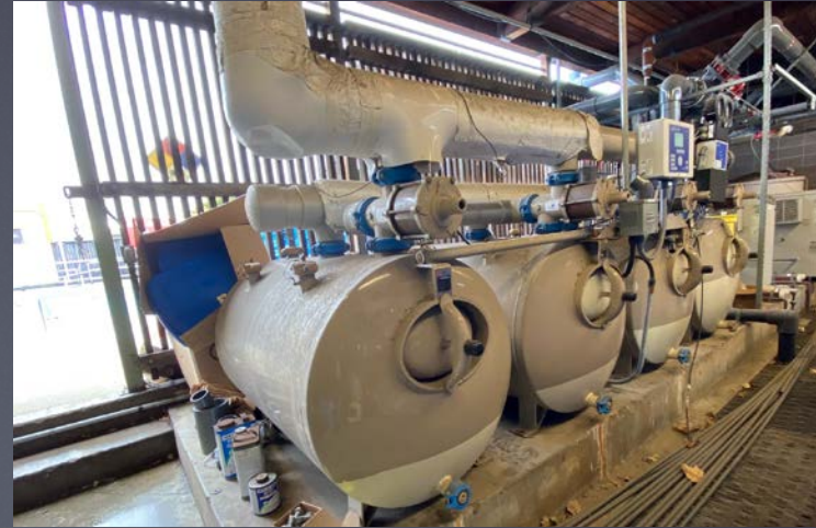
West Campus Pool Filter
