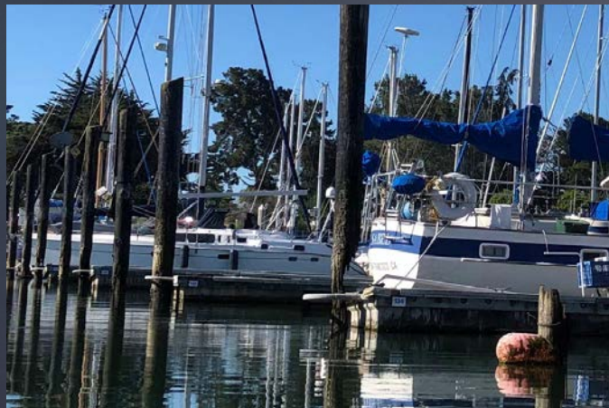
Decaying Timber Piles
