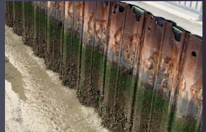
Aged Sheet Pile Wall – South Cove
