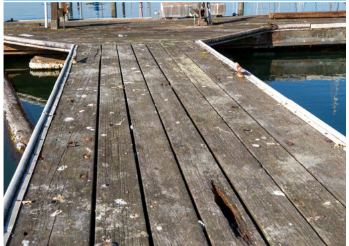
Deteriorated Marina Dock
