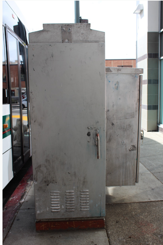
Location: Allston Way/Shattuck Ave.
