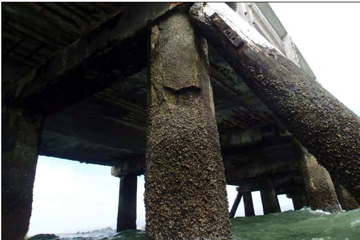
PHOTOGRAPH 16: Pile 403C, open spall
