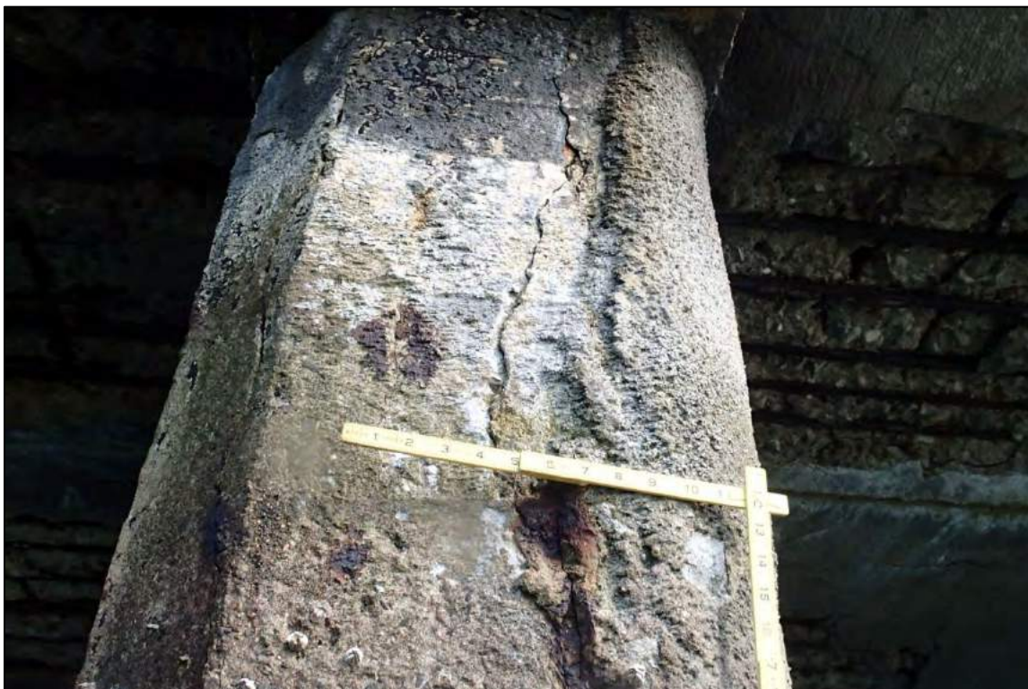
PHOTOGRAPH 12: Pile 408C, closed spall
