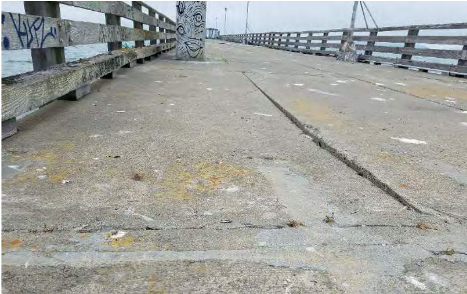
Photo 3-3: Severe Deflection at Section 2 Panel
