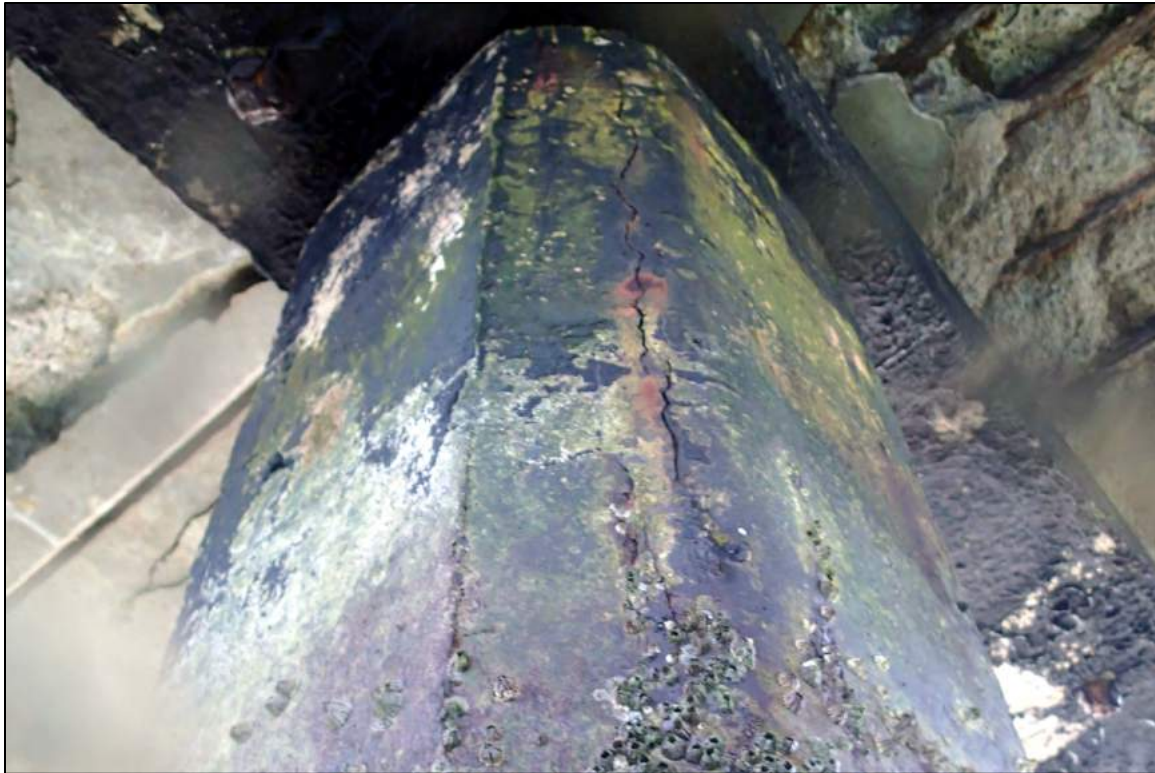
PHOTOGRAPH 9: Pile 304C, vertical crack wider than 1/4 in.
