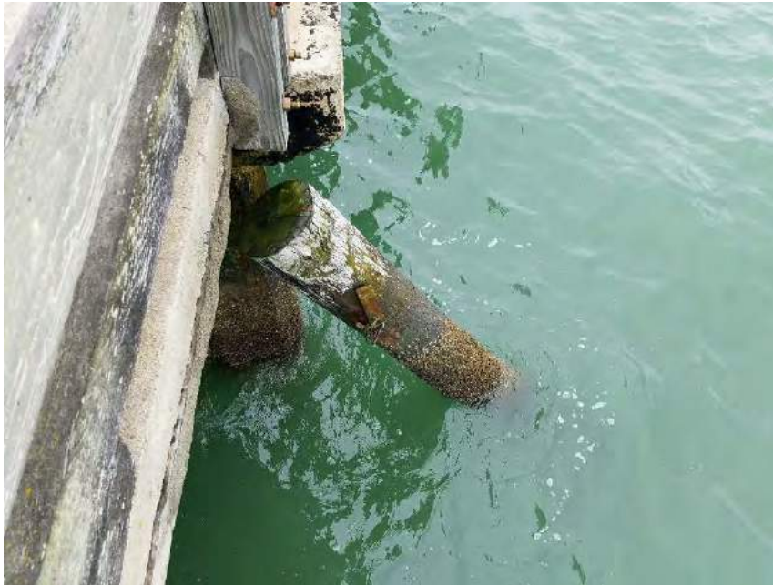
Photo 3-13: Timber Pile Disconnected from Bent Cap
