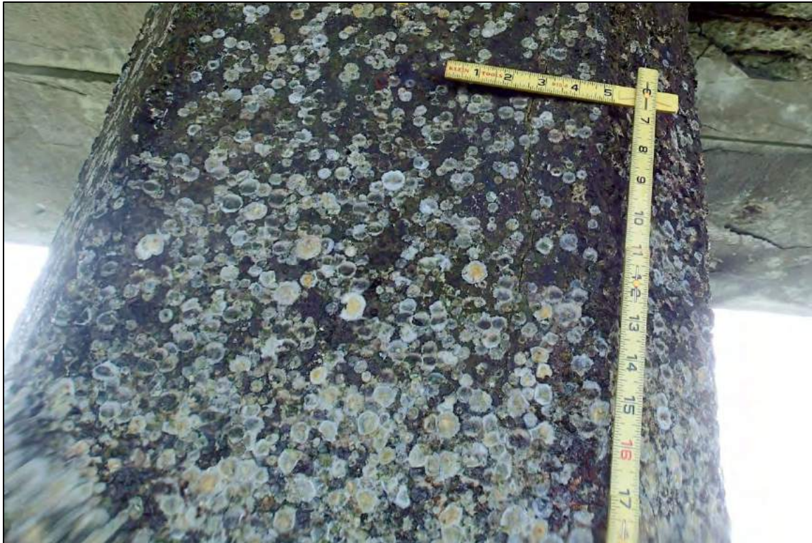
PHOTOGRAPH 7: Pile 423B, vertical crack less than \frac{1}{4} in. wide (Tidal Zone Level II)
