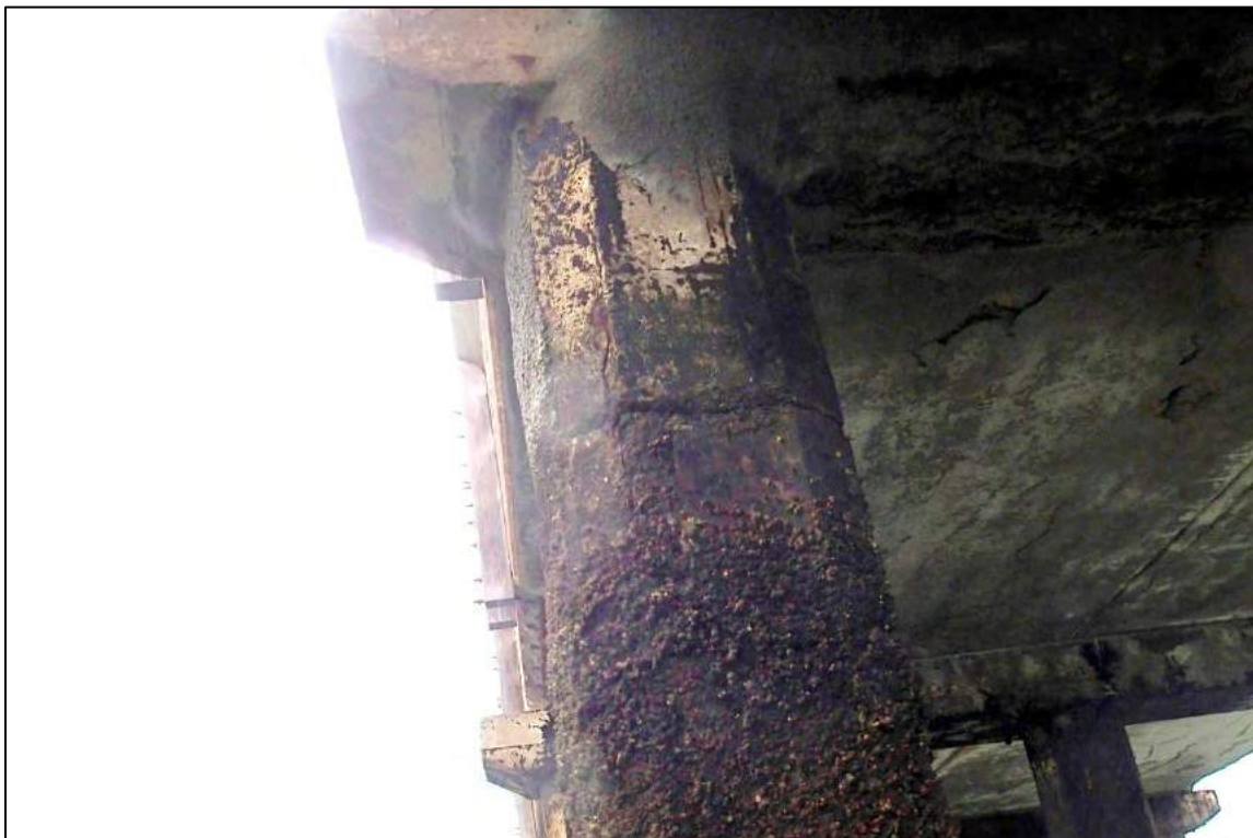
PHOTOGRAPH 18: Pile 301C, horizontal crack
