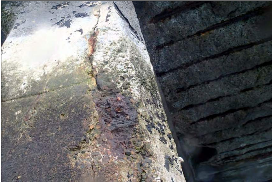
PHOTOGRAPH 15: Pile 339C, open spall
