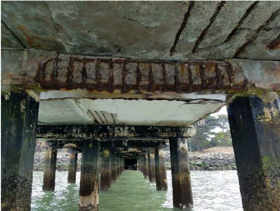
Photo 3-9: Example of Bent Cap with Open Spall in Section 1
