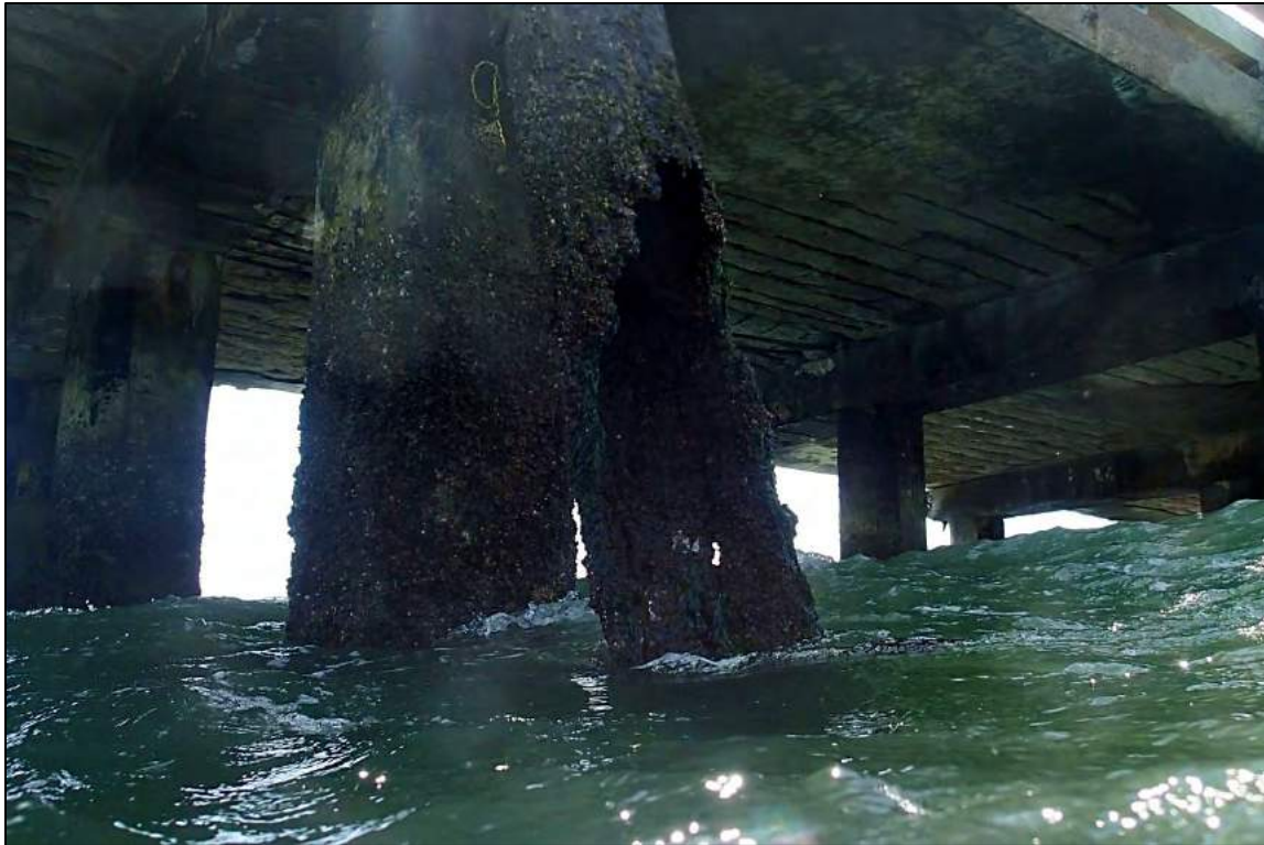
PHOTOGRAPH 23: Pile 376A-BATT, Severe section loss from marine borer
