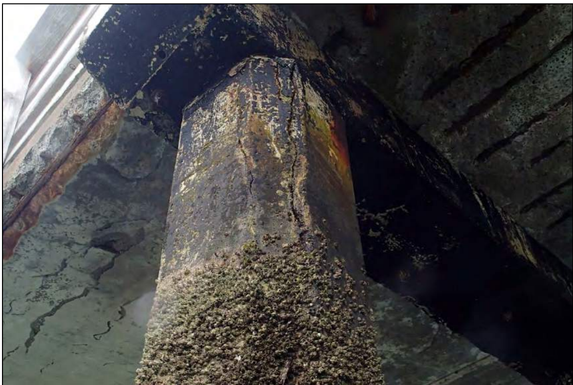
PHOTOGRAPH 10: Pile 303A, closed spall
