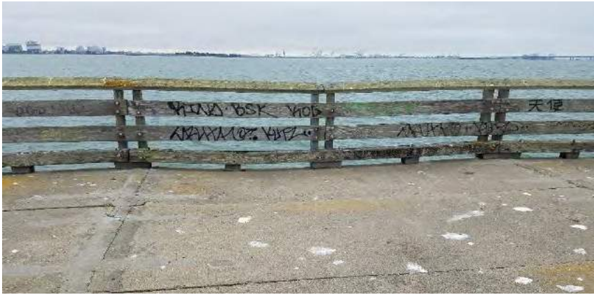
Photo 3-14: Deformed Guardrail Due to Concrete Deflection
