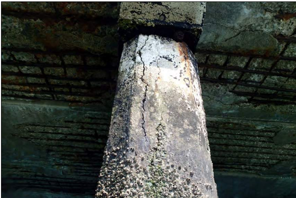
PHOTOGRAPH 14: Pile 445C, closed spall
