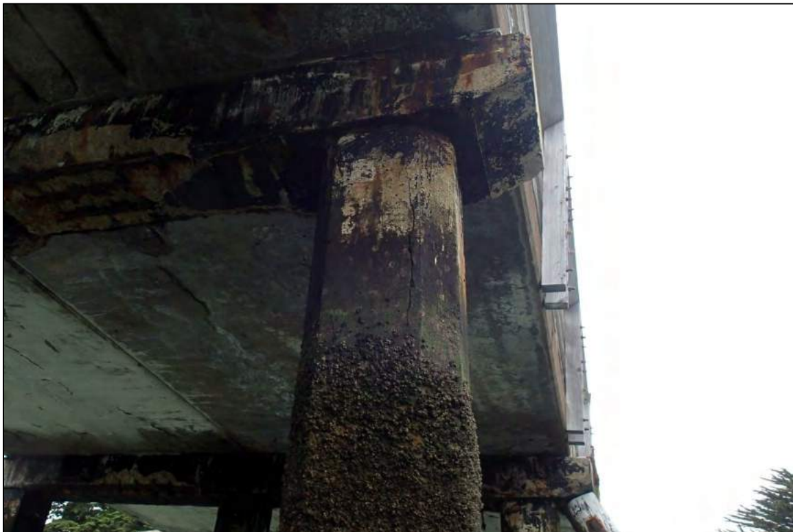
PHOTOGRAPH 2: Pile 287C, vertical crack ¼ in. wide
