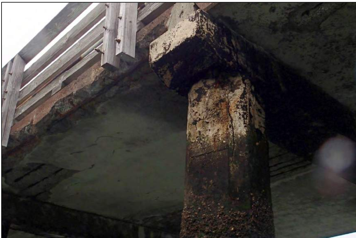
PHOTOGRAPH 8: Pile 289C, vertical crack wider than \frac{1}{4} in.
