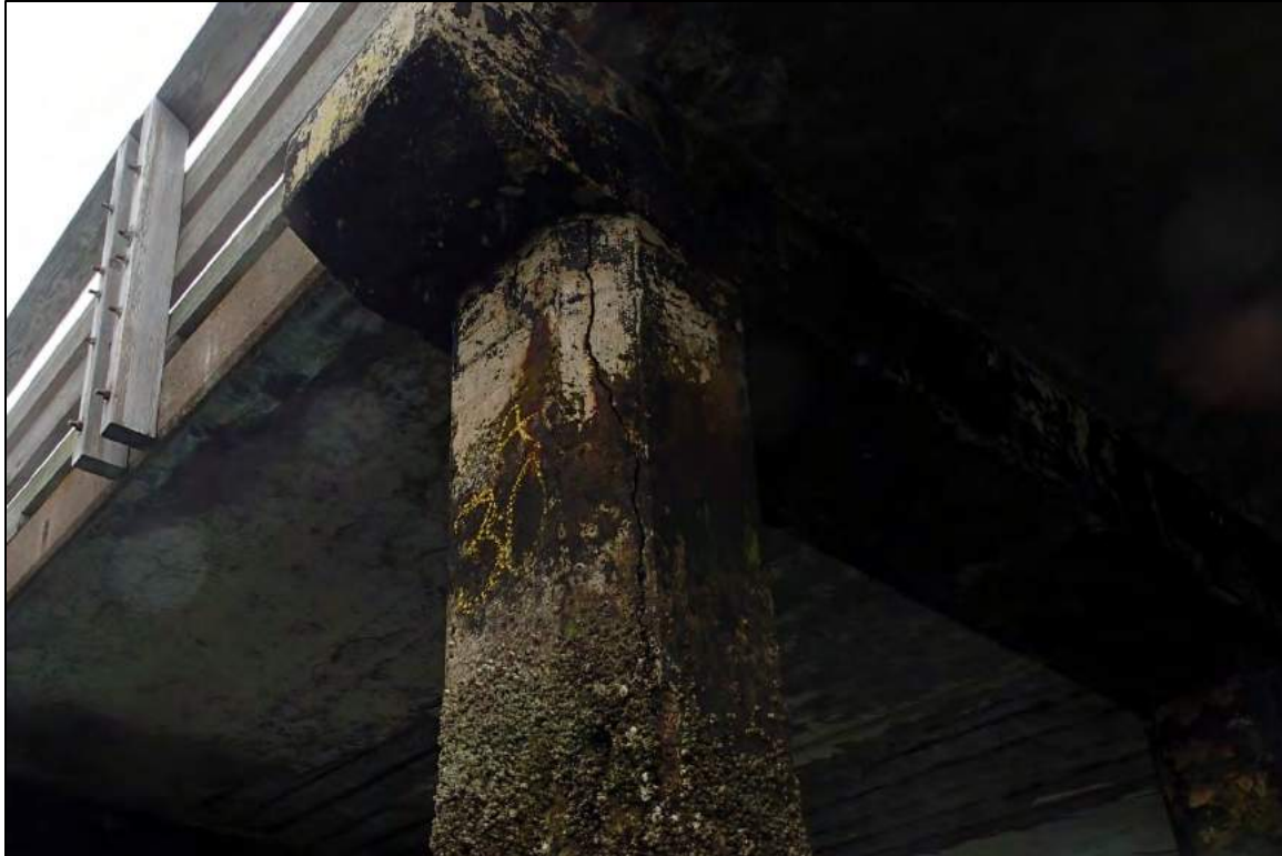
PHOTOGRAPH 11: Pile 311A, closed spall
