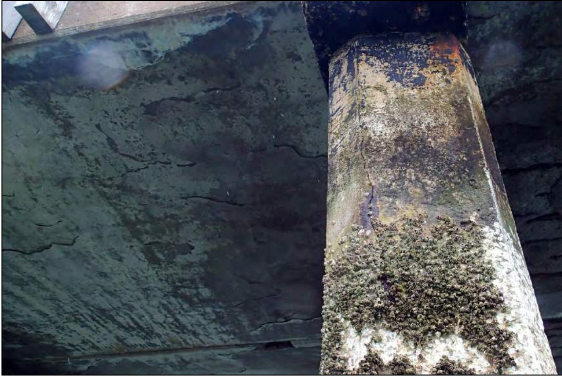
PHOTOGRAPH 3: Pile 306A, vertical crack less than \frac{1}{4} in. wide
