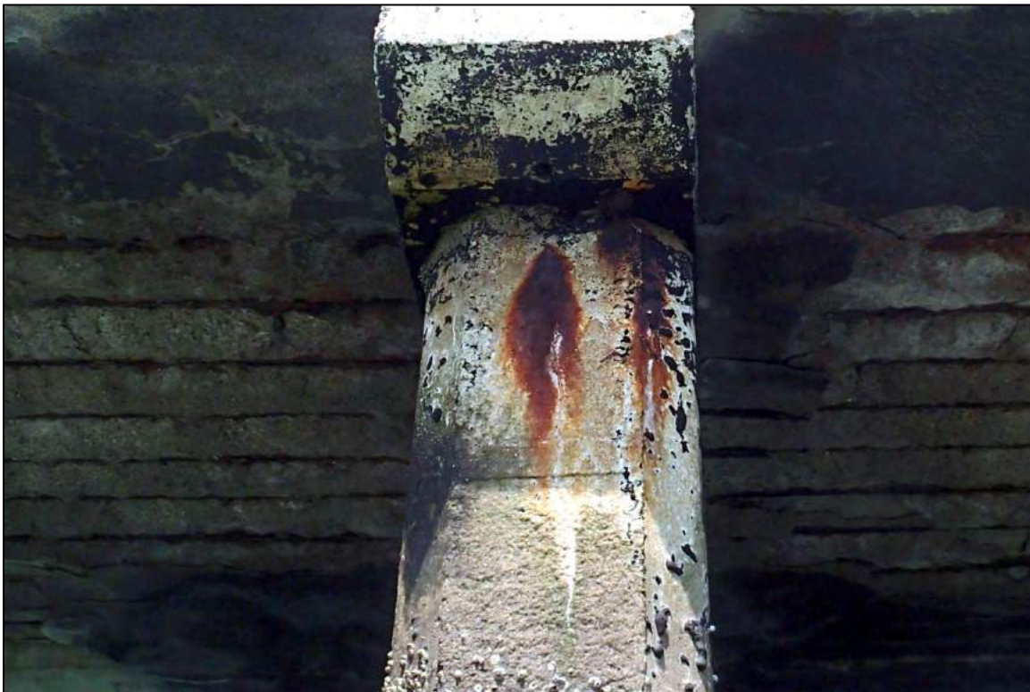
PHOTOGRAPH 4: Pile 379C, vertical crack less than \frac{1}{4} in. wide with corrosion staining and efflorescence
