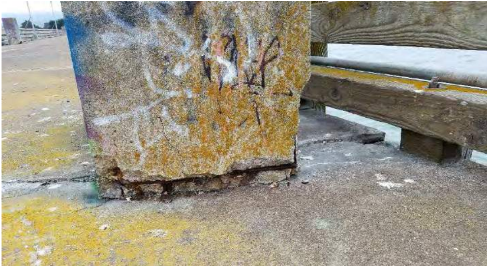
Photo 3-16: Typical condition of bench with concrete spalls
