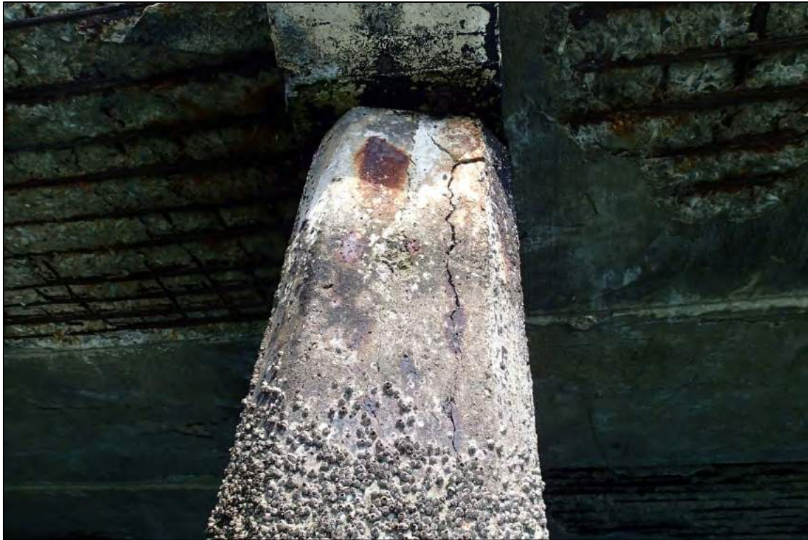
PHOTOGRAPH 13: Pile 443C, closed spall
