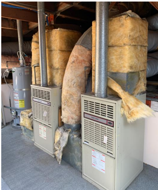
Figure 15: Furnaces at mezzanine floor.
