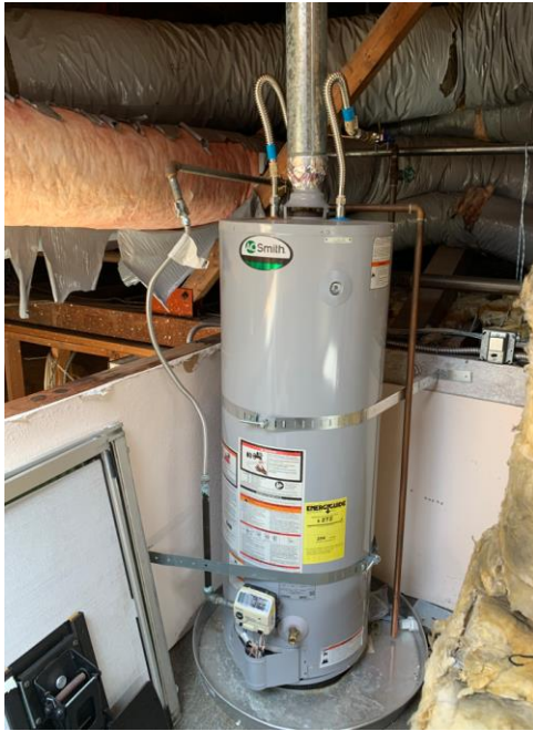
Figure 14: Restrained water heater at mezzanine floor
