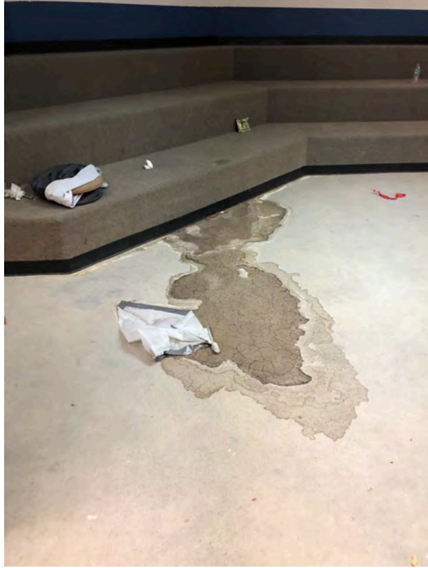
Photograph 11: Staining from ceiling leaks in basement suite.
