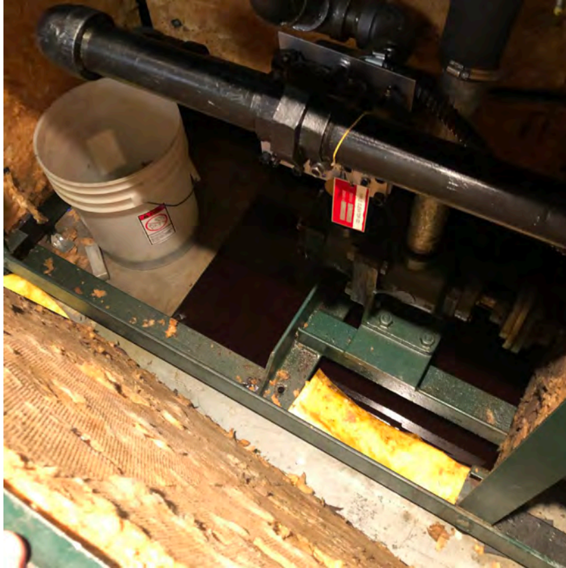
Photograph 9: Standing hydraulic oil in elevator room.
