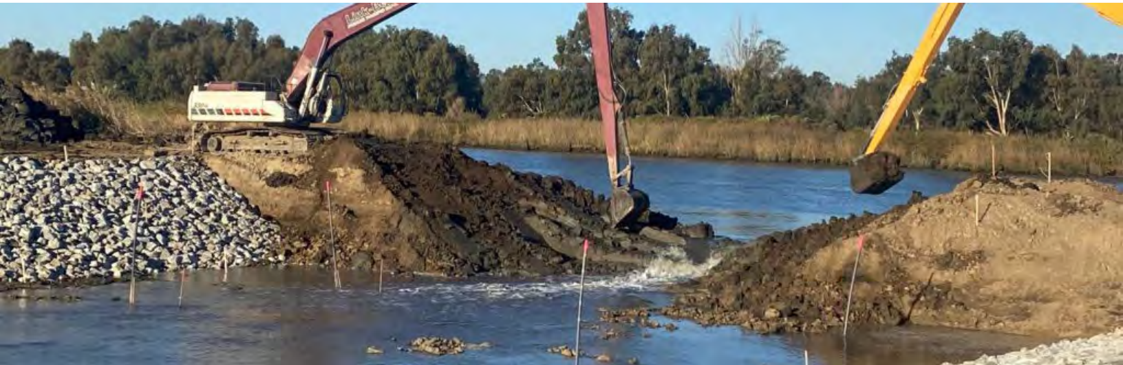
Levee breach in the Montezuma wetlands restoration project. Photo courtesy of the Montezuma wetlands project.
