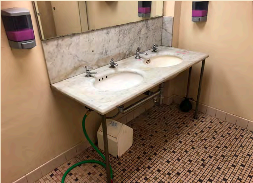
Figure 6.24 Original double marble sink on metal pedestal legs with claw feet located in the first floor Women's Toilet Room.
