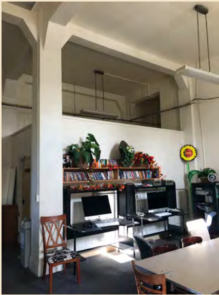
Figure 7.20 Infill walls at the south wing are not full height in the space, allowing the open nature of the original space and the concrete ceiling and beams to be expressed.
