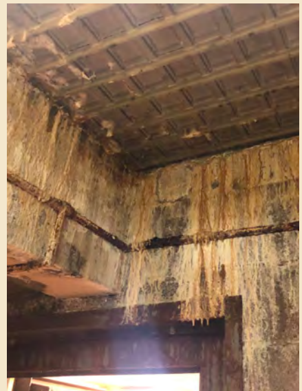
Figure 7.13 The original sidewalk lites of the front entry terrace were poorly infilled with concrete. Salt laden water infiltration has built up over time on the concrete surfaces and electrical conduit below the entry terrace, creating a dangerous condition.
