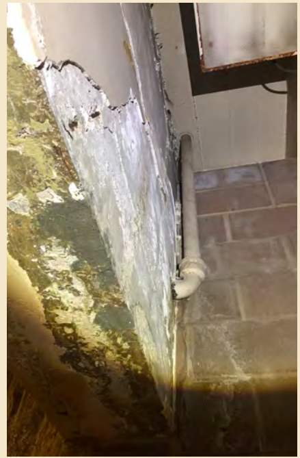
Figure 7.12 Excessive water infiltration at this overhead concrete beam in the basement has caused ferric jacking at the rebar and widespread efflorescence.
