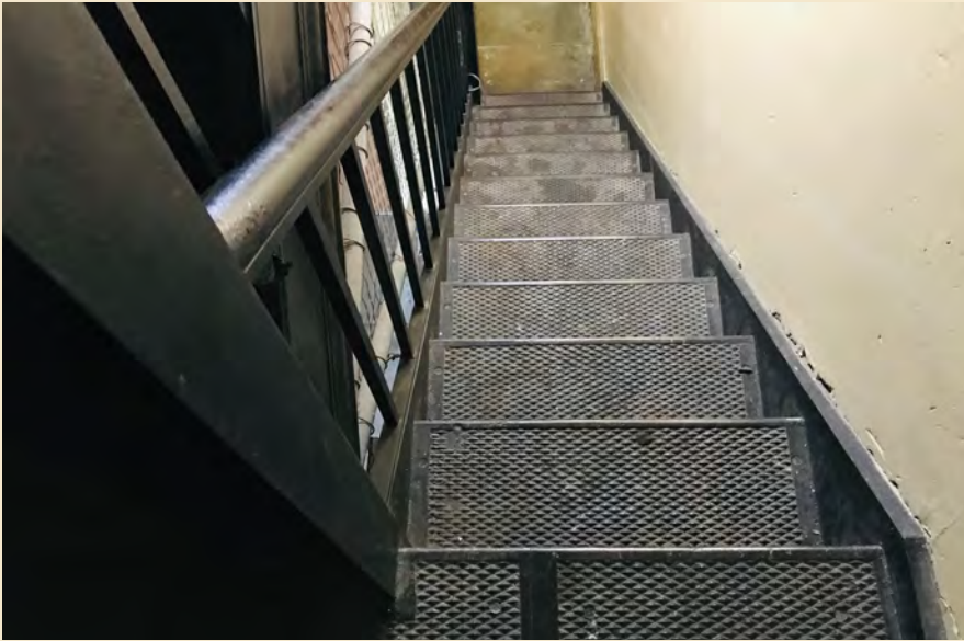
Figure 7.24 The cast iron stair to the second floor is original but does not meet current building code standards.
