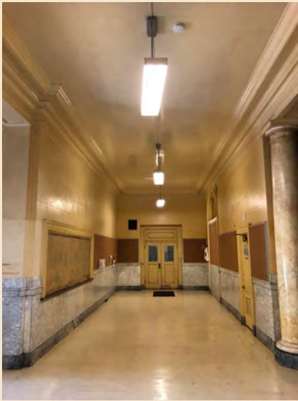
Figure 7.15 Although the original layout and materials of the main entry corridor remain, a number of alterations have altered the appearance and feeling of the space.
