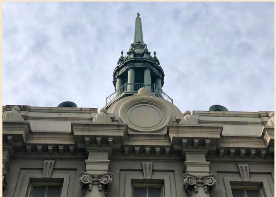
Figure 6.6 The octagonal cupola and spire are made of sheet metal on a wood frame.
