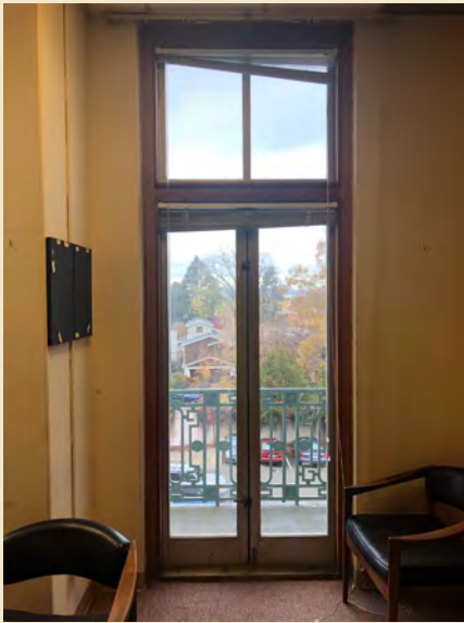
Figure 7.8 At the second floor south wing, the double hung wood windows have been replaced with inappropriate aluminum casement windows.
