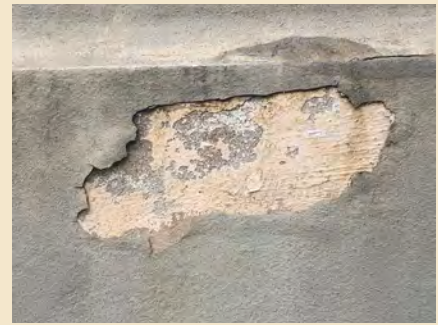
Figure 7.5 At this location on the east elevation, exterior wall coatings have peeled away indicating the many layer of coatings over time.
