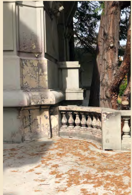
Figure 7.9 A fire started at the north alcove of the entry terrace has damaged the building's exterior finishes.
