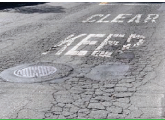
Street surface in need of repairs
