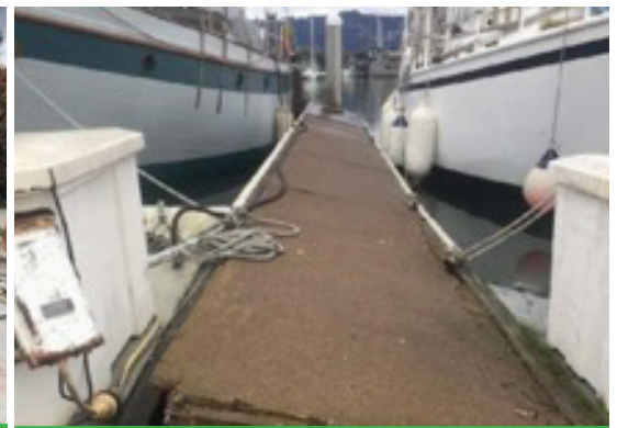
Marina dock in need of repairs
