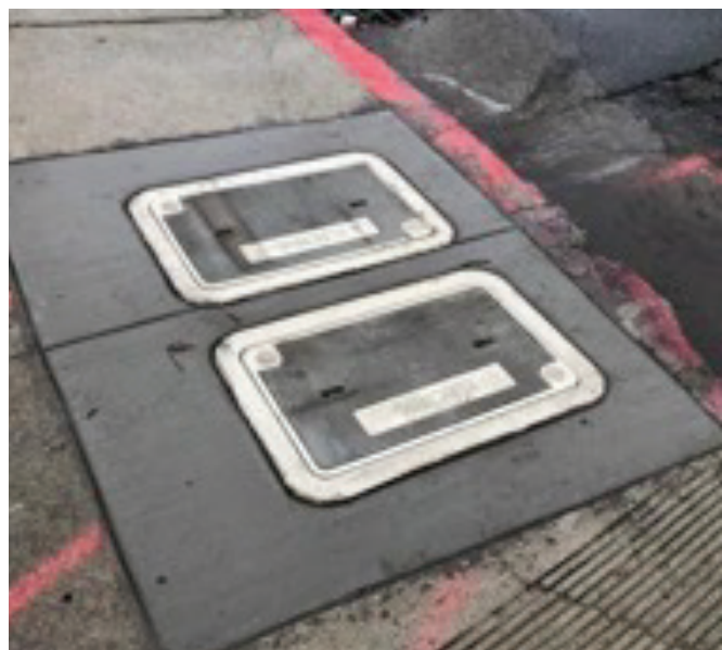
Sidewalk hazard repaired
