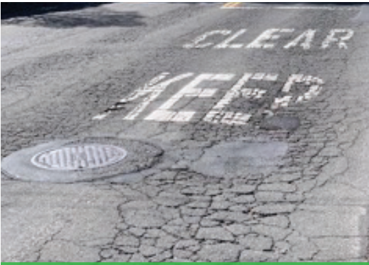
Street surface in need of repairs
