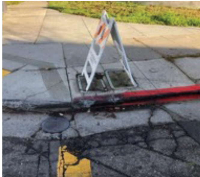
Sidewalk tripping hazard
