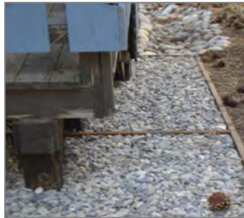
Gravel area under a gutterless roof
