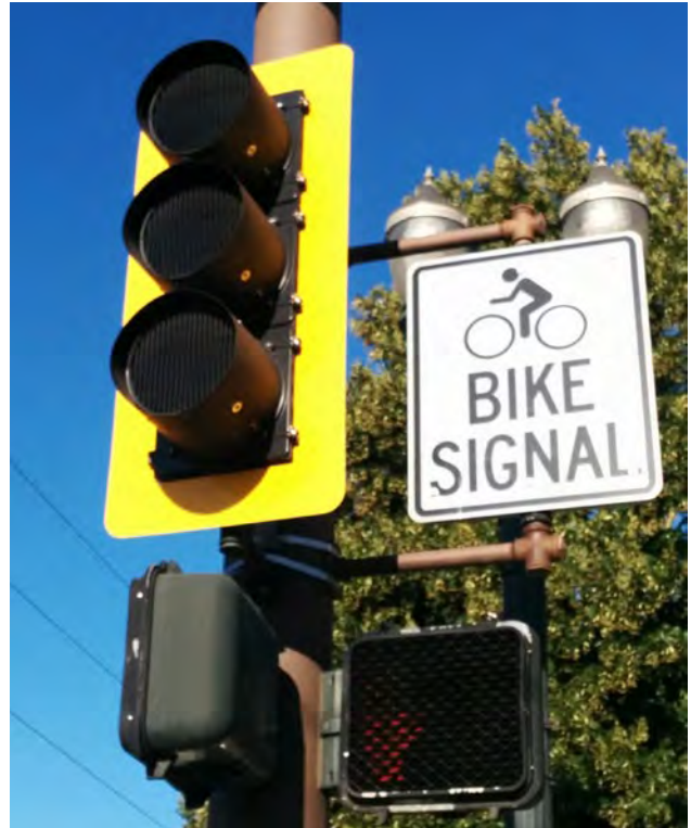
Signal louvers or visibility-limited signal faces reduce the likelihood of motorist in adjacent travel lanes mistaking the bike signal indication with a circular or arrow indication for their travel lane
