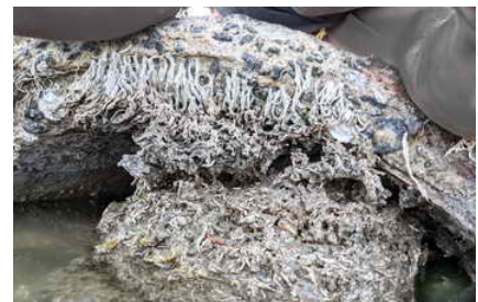
Dead tube worms still block a disused culvert.
