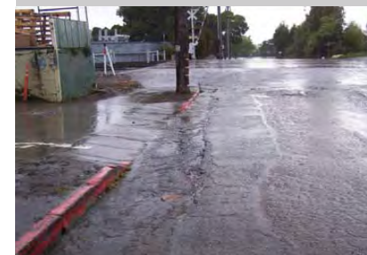
Figure g.2. Downstream Flooding. Green Infrastructure can retain rainwater, and become part of strategies to reduce flooding downstream.
