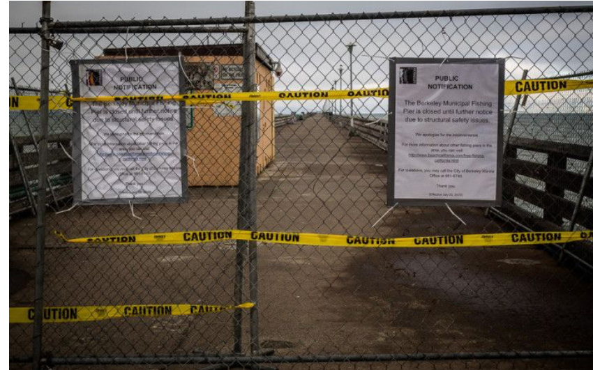
The pier is an example of deteriorated and unsafe infrastructure. Photo: Dorothy Brown
