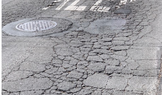
Impervious, deteriorating surface
