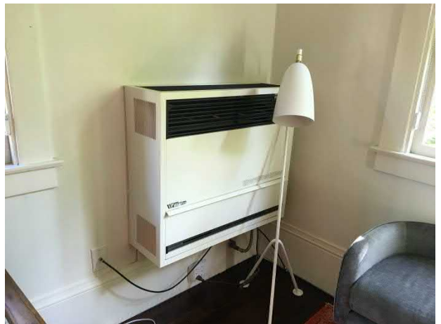
18. Interior view of a wall-mounted heater
