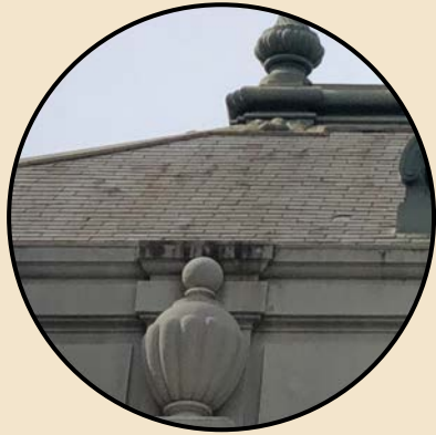
Inappropriate building material
