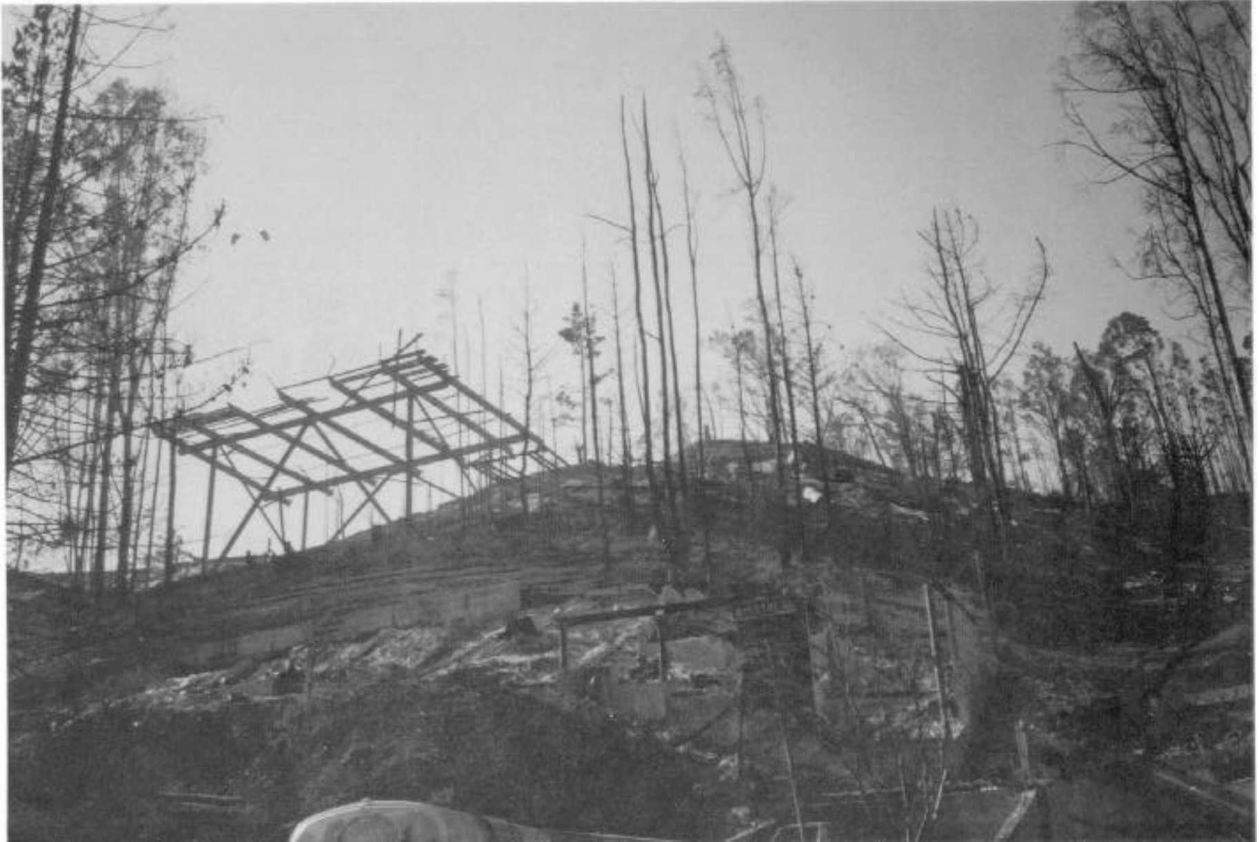
All that remains of one hillside home is the steel supporting structure for the main floor.
