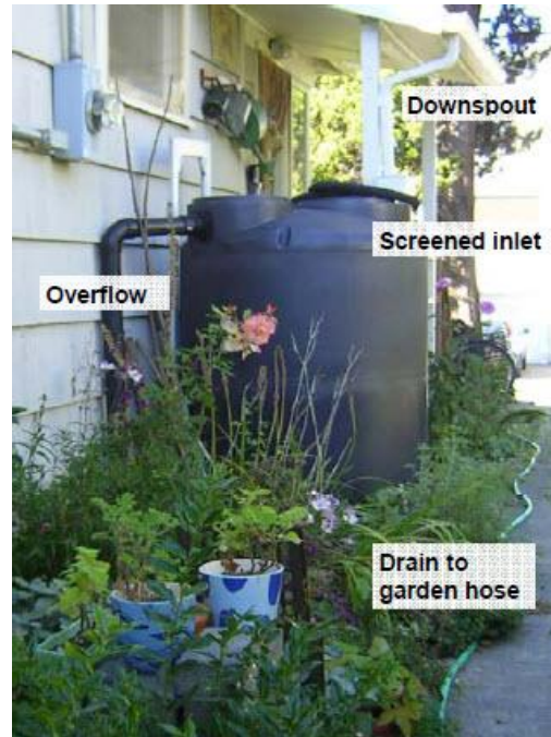
Figure 3-3, Residential Cistern, Seattle
