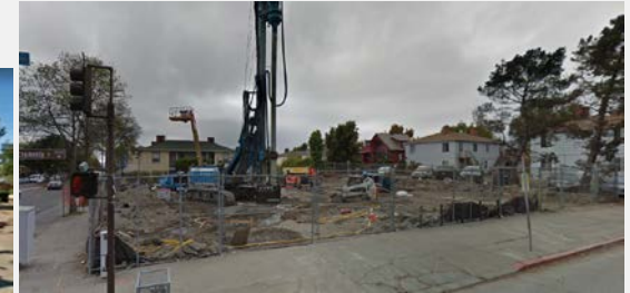
Images: Google Maps Street View Nov 2007 (left) and construction underway in October 2017 (right).
